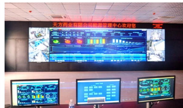
Topfond Pharma Co Ltd under Genertec Meheco introduced advanced domestic technology and equipment, and successively built a high-standard wastewater treatment stations (automation control centers), an exhaust gas treatment system, and an automation energy dispatch center, so as to develop circular economy and gradually realize the goal of "energy-saving by power reduction, electricity-saving through fermentation, and energy recycling".
